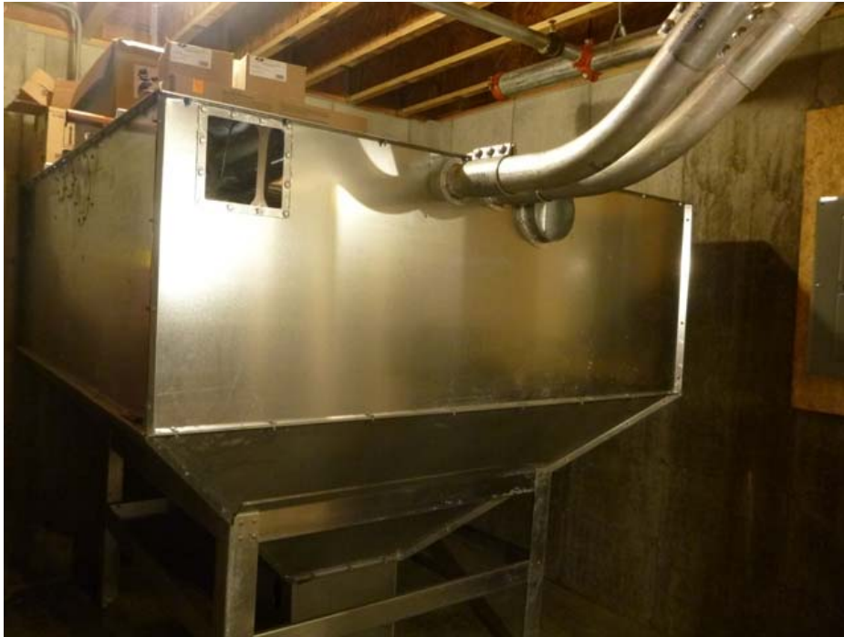
(Figure 3: Indoor pellet storage bin with pipes)
